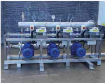
Three-pump Hydrovar booster set, complete with a PLC and HMI.
