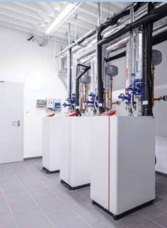
Heat pump room in modern commercial building
