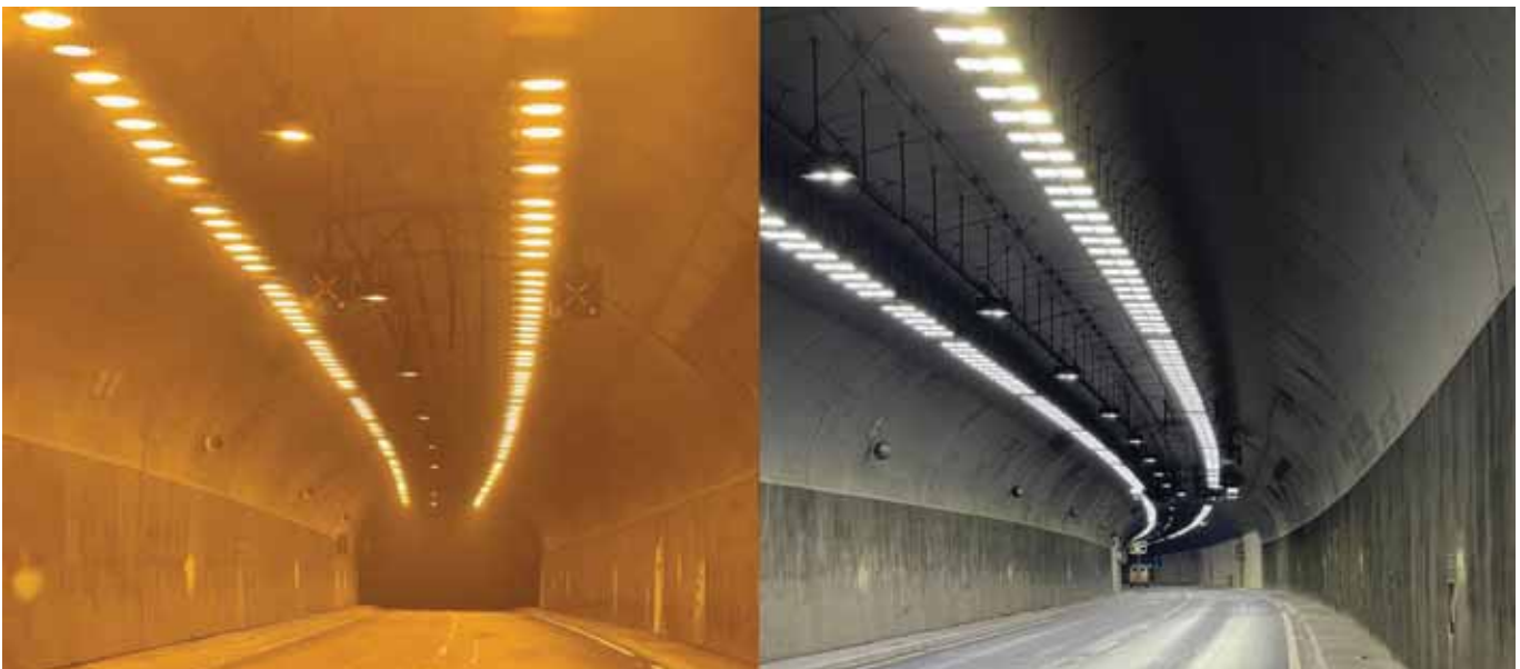
Dublin Port Tunnel before (left) and after (right) the LED upgrade.
