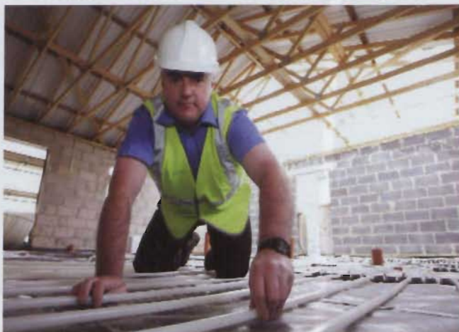
Paul van de Woning of the Myson Floortec team, supervising a home installation.
