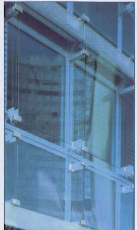
Traditional Climate Facade 2 — external brise soleil and external sacrificial pane of glass, note the gaps around the pane to allow the entire skin to ventilate
