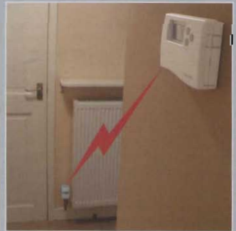
In a CM Zone system, wireless time/temperature controls are sent to each radiator
