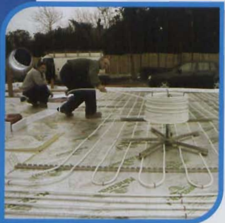
Unipipe underfloor heating
