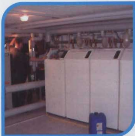
120 kW NIBE Ground Source Heat Pump Installation
