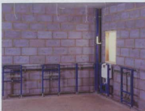
Each Geberit Duofix frame can be installed quickly and easily. Shown here with system rail, the elements are fixed to two rails, secured to the wall and floor. Water supply and drainage can easily be installed and connected.
