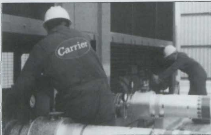
Core's engineers are trained to commission, troubleshoot and maintain both Carrier and Liebert products. The company is also a member of the Refrigeration Service Engineers Society (RSES)
