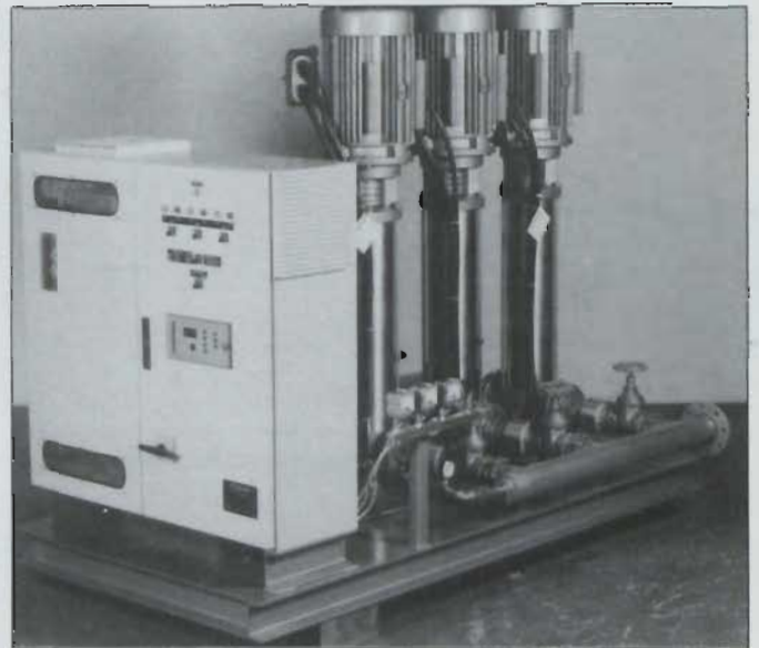
Holpak 3-pump variable speed packaged pumpset, as designed and manufactured exclusively by Holfeld Pumps. This particular unit is installed in a high-profile international hotel in Dublin. Contact: Alison Kirwan, H R Holfeld (Hydraulics) Ltd. Tel: 01 - 288 7361.
