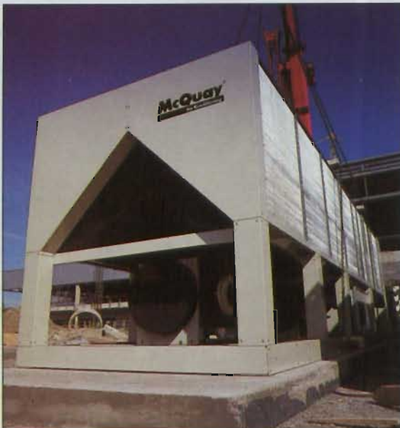
ABOVE: McQuay International single screw chiller from Thermo Systems
