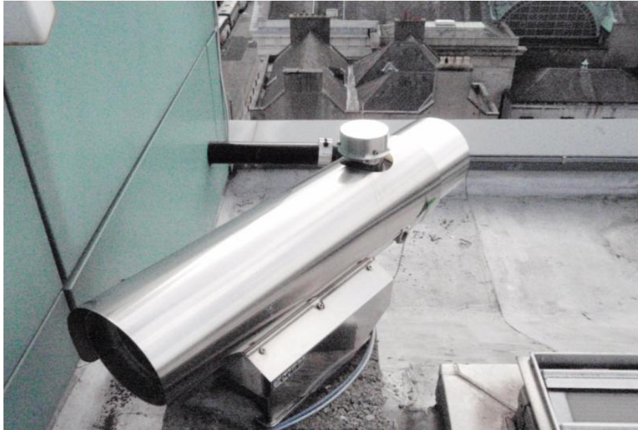
Figure 2.9 OPSIS system emitter housing on the roof of DIT Cathal Brugha Street
