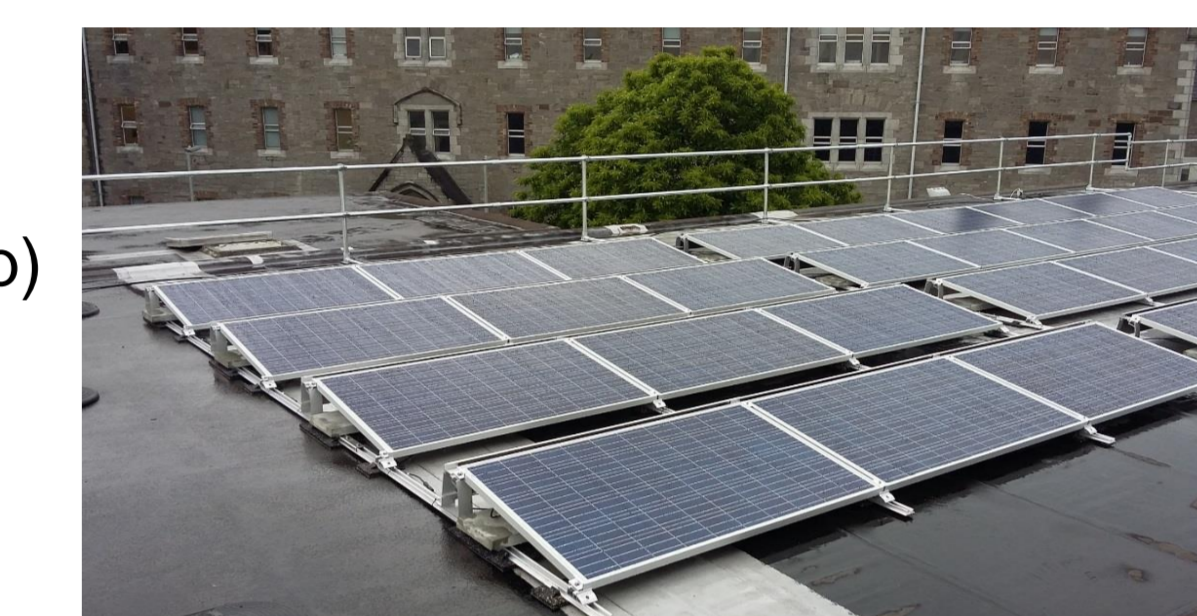
Figure 5. PV array of 42 modules located on a roof
