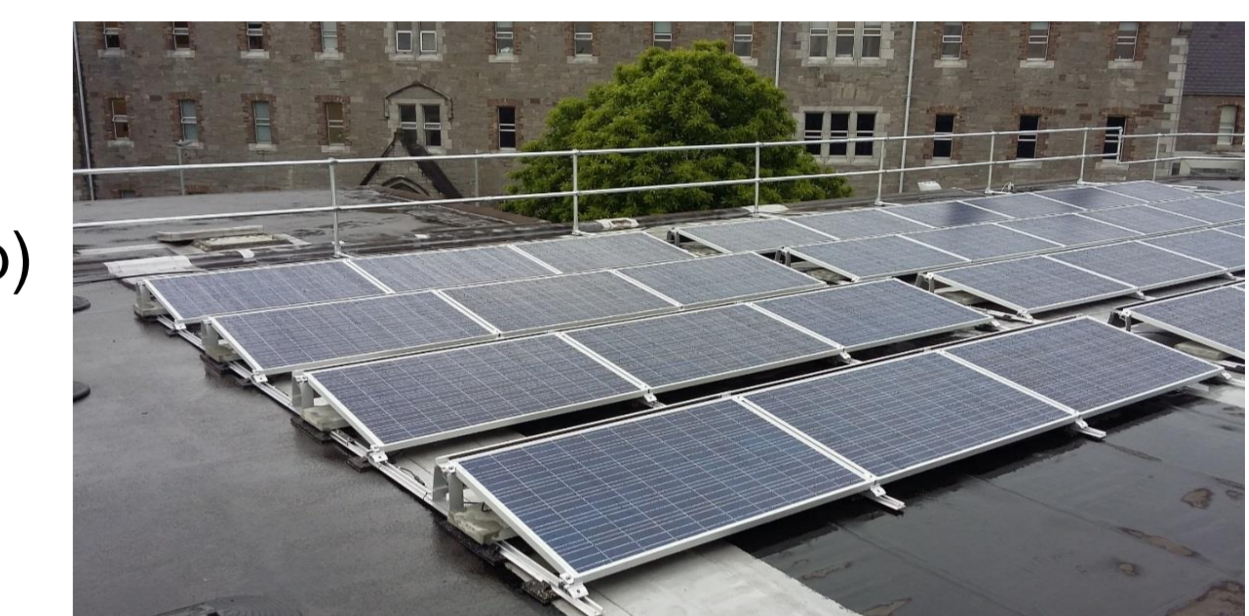
Figure 5. PV array of 42 modules located on a roof
