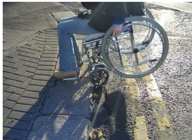
Figure 2. Wheelchair user trying to mount a pavement without a kerb cut
