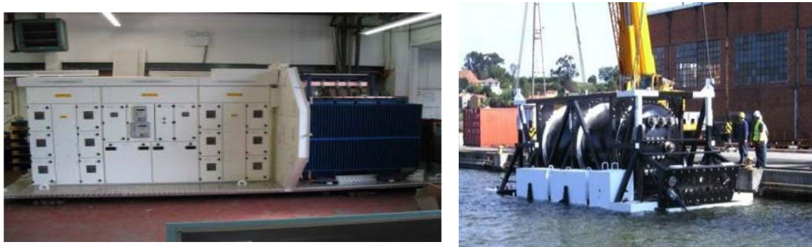
FIGURE 3.15 OPTS UNDERWATER SUBSTATION POD – 1.5MW CONSTRUCTION AND TEST DEPLOYMENT (COURTESY OCEAN POWER TECHNOLOGIES)
