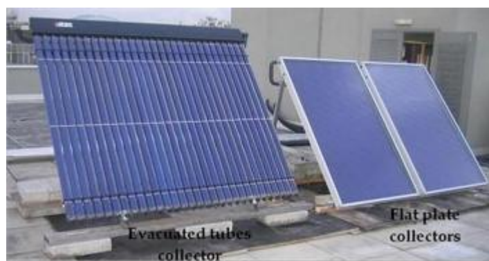
Figure 5.10. The solar thermal systems built and installed at a site in Dublin [63].
