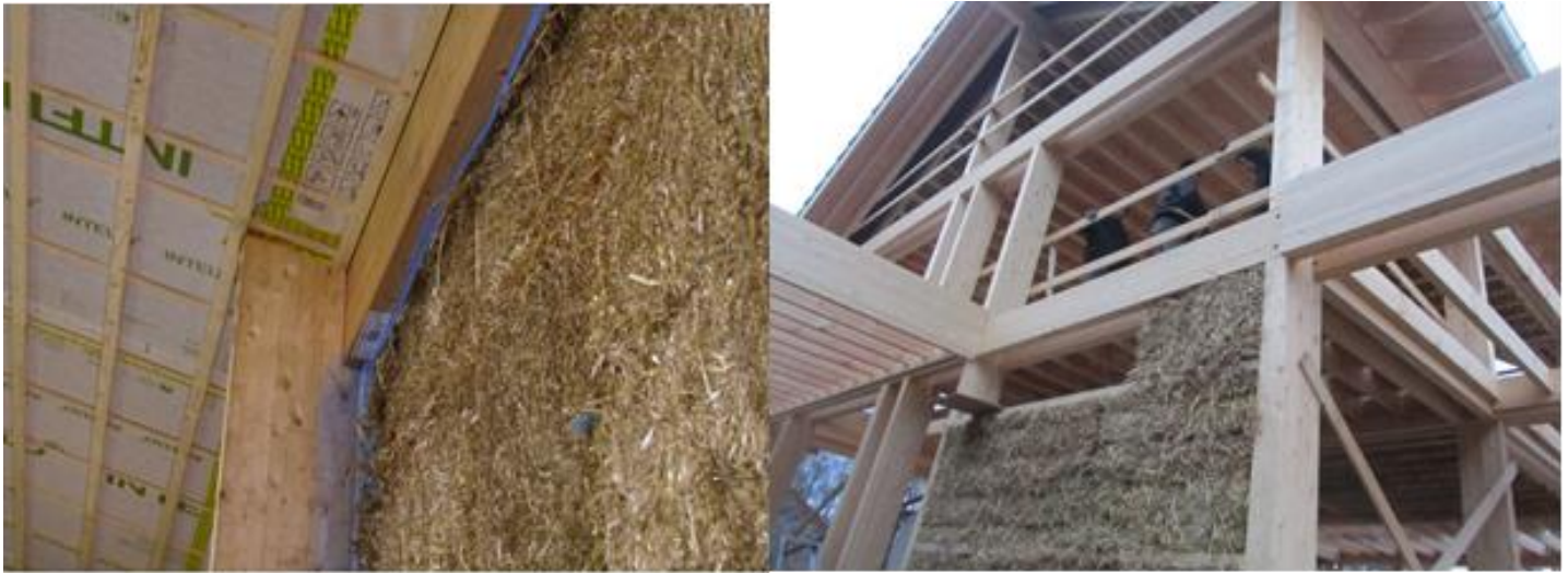
Figure 7: Showing examples of straw application of straw bale as infill wall in timber post and beam construction. Architecture barchi Belgium [Source Author].
