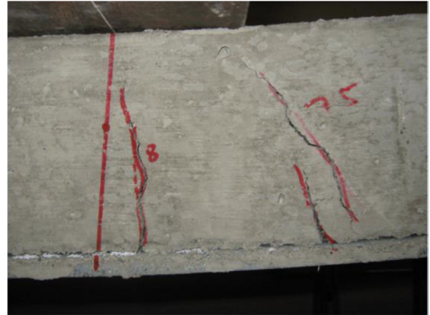
Diagonal Shear cracks – Right hand side
