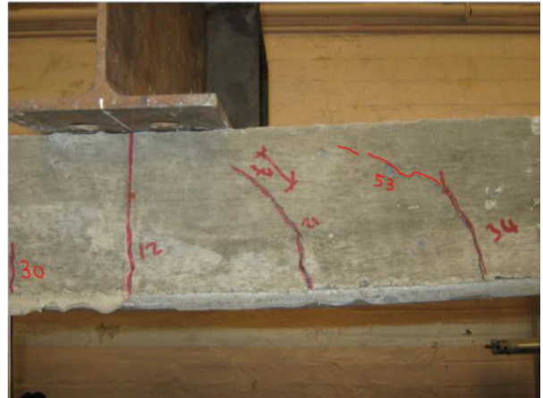
Diagonal Shear cracks – Right hand side
