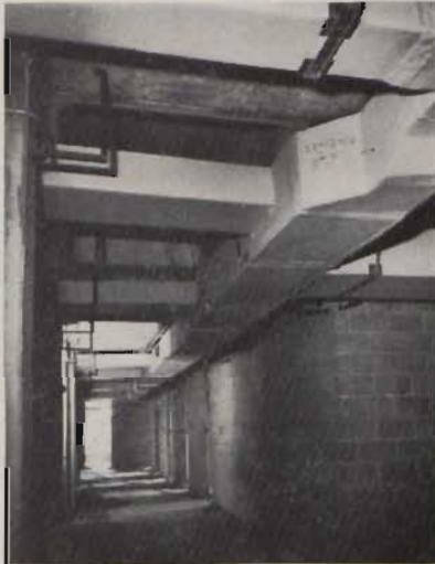
● The illustration shows a return air duct in one of the corridors. Branches are connected to return air grilles in a series of classrooms.
