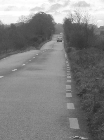
Figure 3. Extreme undulations on N62 rampart road, County Offaly, Ireland.
