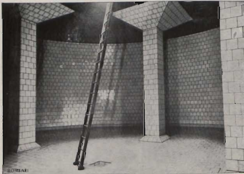
UNDERGROUND FUEL OIL STORAGE TANK 70,000 GLS. (DUBLIN)
