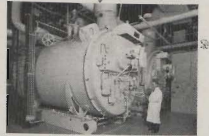
Two Marshall CB400 Automatic boilers
