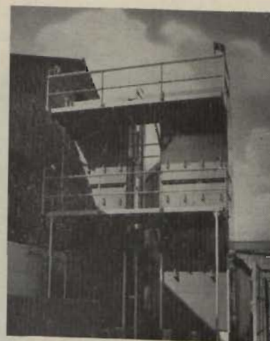
● Front view of twin test evaporative water cooling towers.
