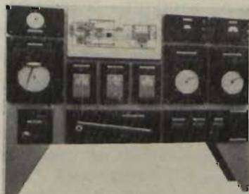
● Operating control panel for cooling tower test centre showing mimic diagrams.
