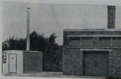
● Our picture shows the Marshall and Anderson packaged boiler house beside the brick boiler house it replaced in a recent installation (see review).
