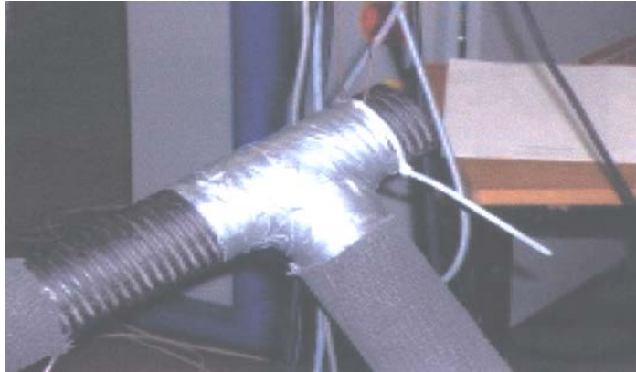
Figure 4: Connection of air condition rig and the intake system
