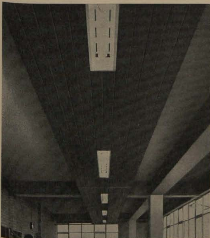
FIG. 2—A recently introduced system which makes it possible to position both radiant heating and lighting in one assembly.
