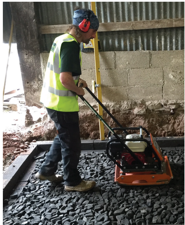
Figure 6 – Construction worker compacting recycled foamed glass aggregate during installation of “Sublime Insulated Limecrete Floor” (image supplied by Tŷ-Mawr Lime Ltd).
