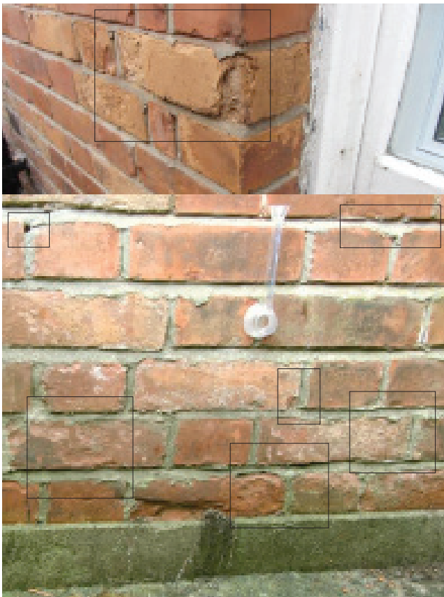
Figure 2 – Damage to brick in case study house: (above) whole brick spalling, (below) loss of brick edge and surface at base of external wall.
