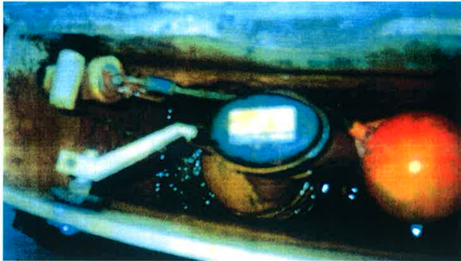
Figure 1.3. Toilet Cistern with Excess Iron in the Water.
