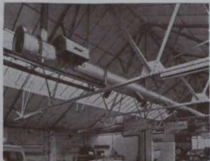
The model X 19 roof mounted heater from the Nu-Way Heating Ltd. range. from previous page.
