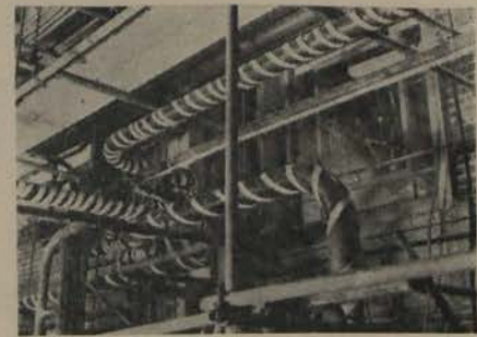
RIGHT —Isotapes, the well-known flexible heating tapes are shown here in use at a power station.
