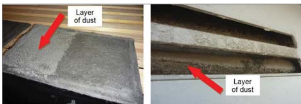
Figure 7: Dirty extract filter (half cleaned for comparison) and clogged up external inlet grille.
