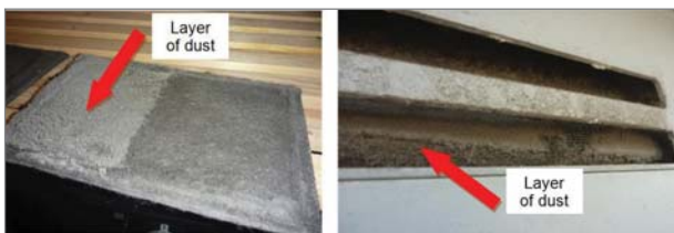
Figure 7: Dirty extract filter (half cleaned for comparison) and clogged up external inlet grille.
