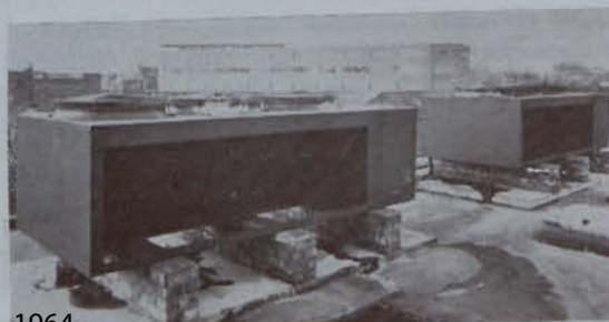
A three-quarter view of the outdoor condenser units of the Thermo-tank heat pump installation at Ilford, Essex.
