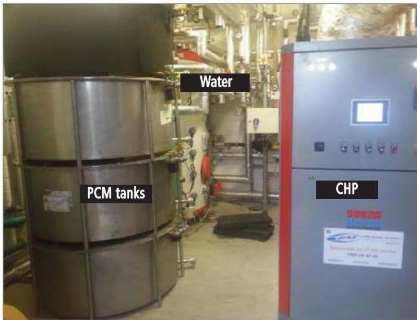
Figure 3: Plant room showing the CHP, PCM tanks and sensible water tank.
