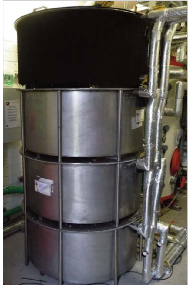
Figure 2: PCM-TES installation during commissioning (only top unit shown insulated).
