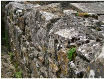
Fig 8. Biological growth on stone wall at Clonmacnoise (C. Daly 2009)
