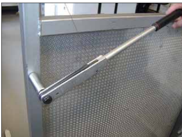
Figure 4.21. Photograph showing application of the torque wrench to the fixing clamps which are fabricated from threaded bars.
