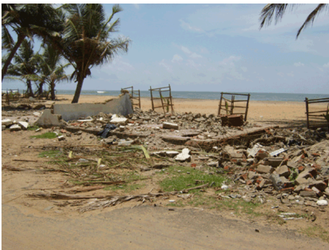
Fig 3 Total structural failure of blockwork homes within coastal zone
