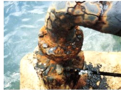
Figure 1. Sea water corrosion damage of a shaft without coating
