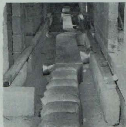
● This is another view of duct run with side take offs. (See also pictures on Page Thirty-four).
