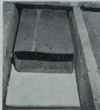
● This picture, taken on the site at Malahide, shows part of the main duct being laid in concrete slab with Aeroboard insulation.
