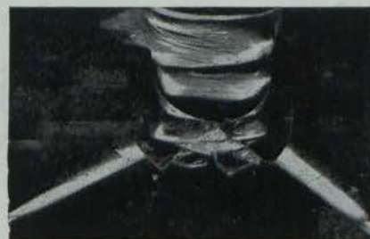
● Part of the main duct (insulated) with branch pipes running under suspended floor.
