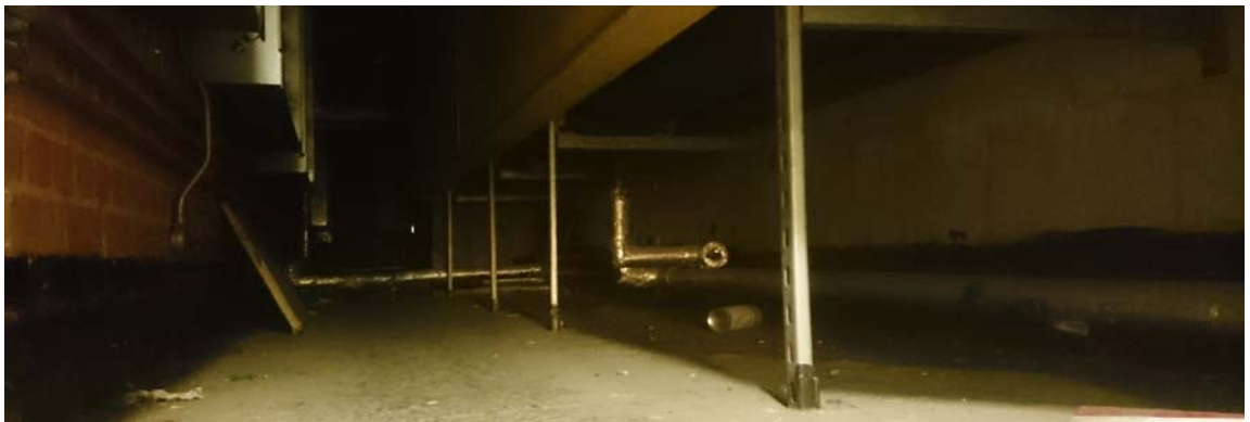
Figure 86: plenum beneath studio theatre space, heating elements below inlet grills in floor
