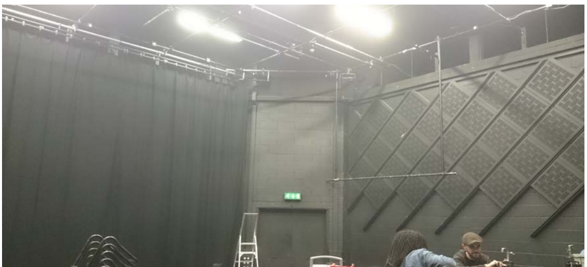
Figure 87: studio theatre space, inlet grills in floor and outlet at top of walls
