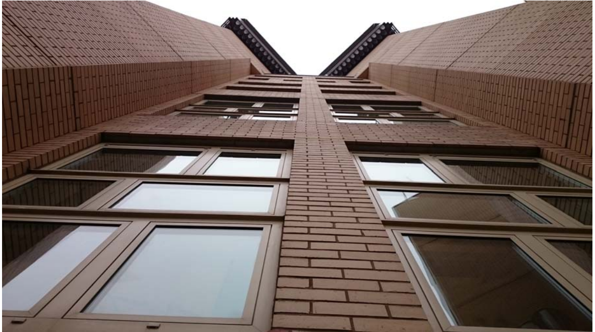
Figure 111: external view between perimeter extract towers showing metal stack terminations from below
