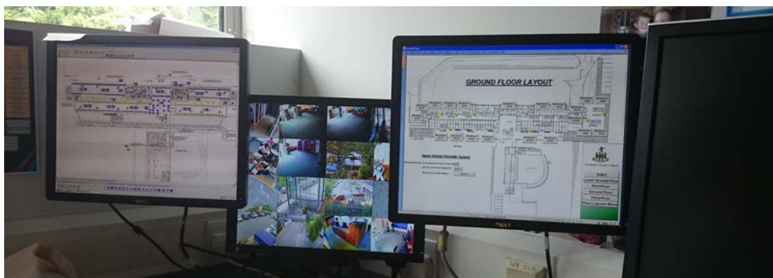
Figure 63: BEMS user interface – monitoring temperature internally and externally, wind direction and speed, ventilation openings.
