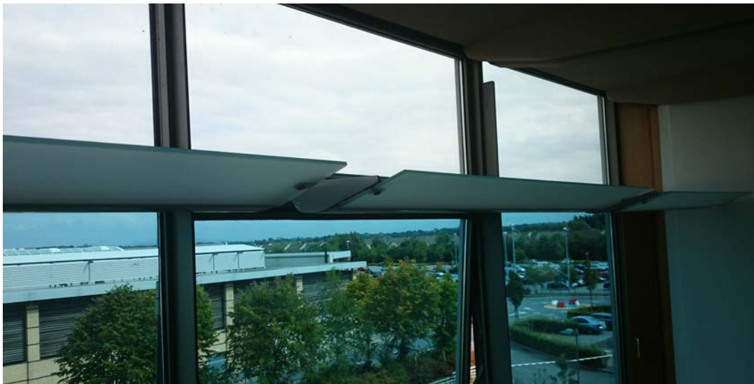
Figure 67: office internal elevation showing light shelves and ventilation shutter and opening window
