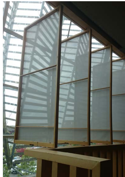
Figure 69: detail of manually operated shutter screen between office and atrium to control daylight levels.
