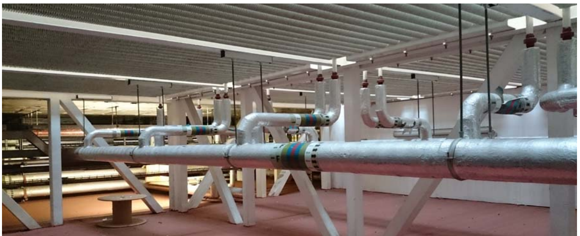
Figure 103: plenum beneath light well/ air ingress and fin heating radiators
