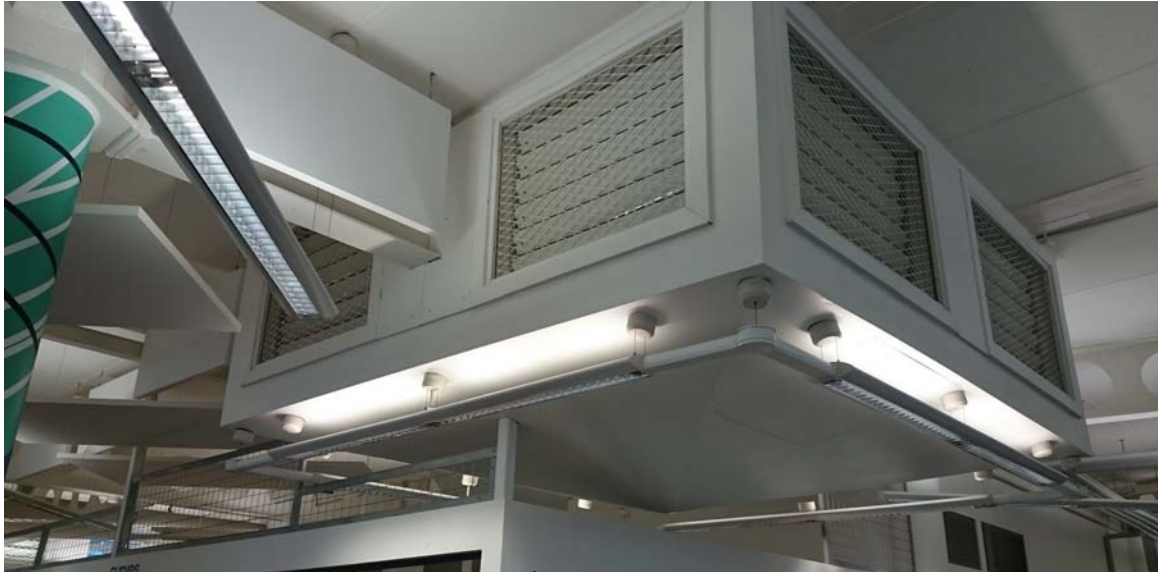
Figure 107: top library floor showing ceiling extract vents
