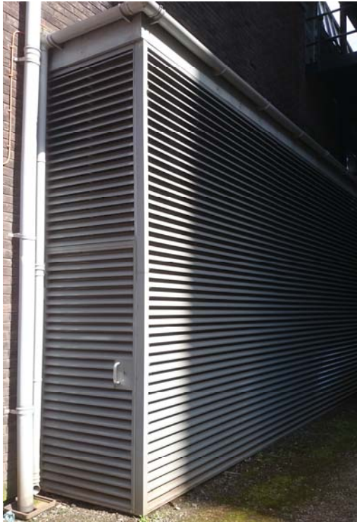
Figure 77: louvered air intake to main theatre space from courtyard
