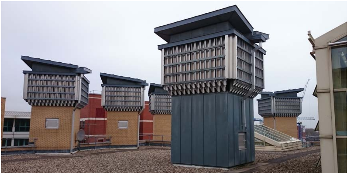
Figure 102: view of extract stacks at roof level – note blue clad stack is for top floor only
