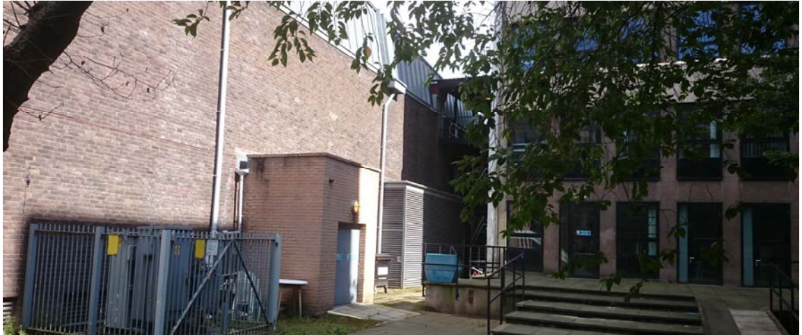
Figure 91: the pedestrian courtyard to the rear of main theatre showing louvered air intake beyond fire escape door
