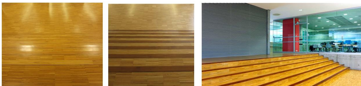
Figure 6 The pictures shows before and after shots of a stairway that has been contrasted. Photo: Statsbygg
