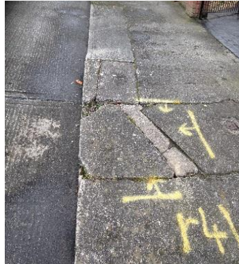
Figure 8: Broken paving on Riverside Avenue
