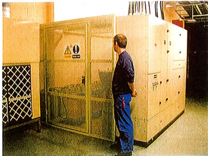
View of Caged Capacitor/Inductor Compound
