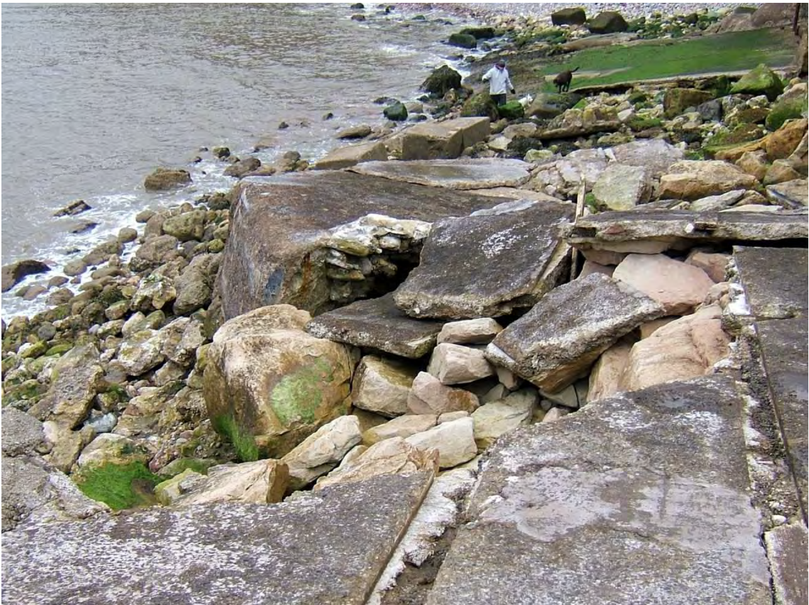
Figure 5.8. Storm damage to modern pier at Boddin Limekiln, April 2012
