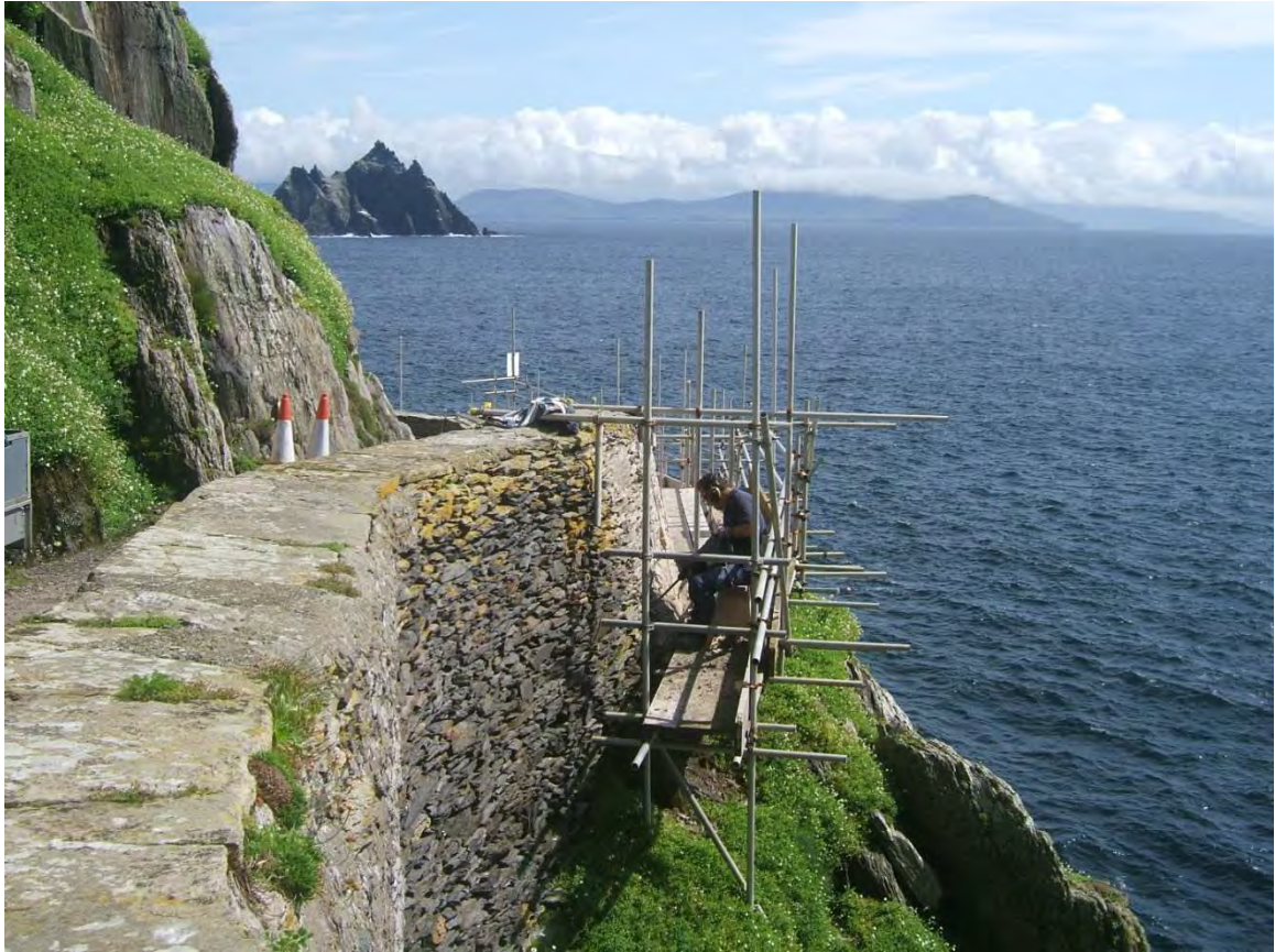
Figure 7.7. Conservation of retaining wall for roadway from pier to monastery steps (Small Skellig visible in background) August 2012
