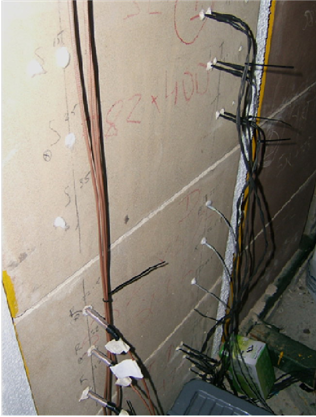
Figure 5.4. Detail of internal face of stone wall showing two types of embedded moisture sensors, February 2012
