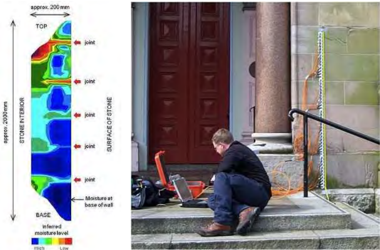
Figure 5.6. Non-destructive 2D electrical resistance tomography (ERT) being used to map moisture distribution within masonry by researchers from the school of Geography, Queens University, Belfast ( www.qub.ie/ )
