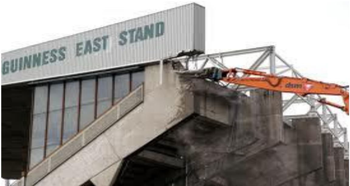
Fig 12 (Below) Demolition of the East stand at the original Lansdowne road stadium. (Source – www.Flickr.com )
