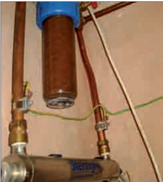
Figure 7: Filter and ultra violet unit.
