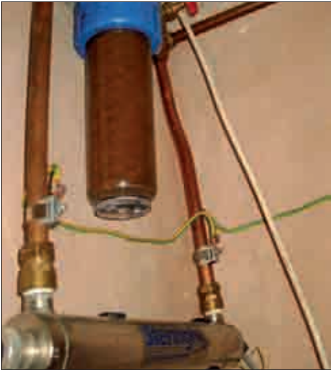
Figure 7: Filter and ultraviolet unit.
