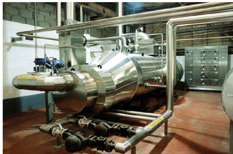
Figure 3.7 Clean Steam Generator and distribution pipework
