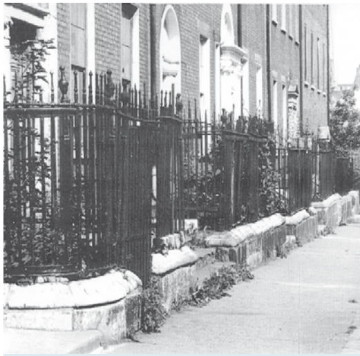
Fig.7.2.1 Detail of railings. The Henrietta Street houses display high quality ironwork that contributes greatly to the streetscape. Specialist technical advice is vital when conserving these important architectural elements. (Photo IAA)
