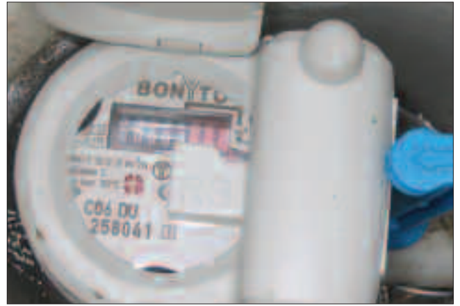
Fig. 2.13 Meter with attached transmitter located externally.
