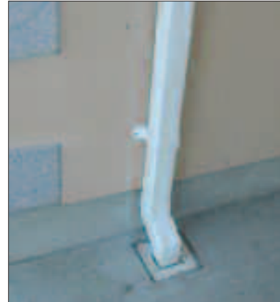
Fig. 2.7 Sealed downpipe to rainwater catchment system.
