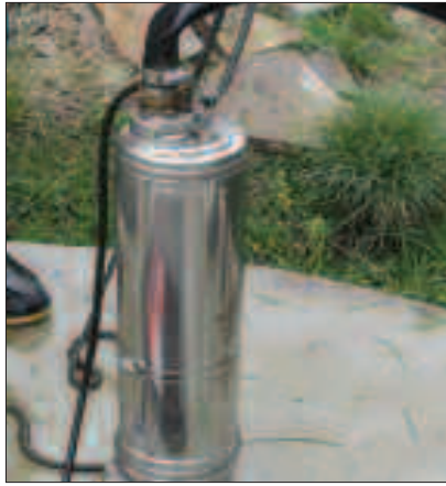
Fig. 2.4 Submersible pump installed in underground rainwater storage tank.
