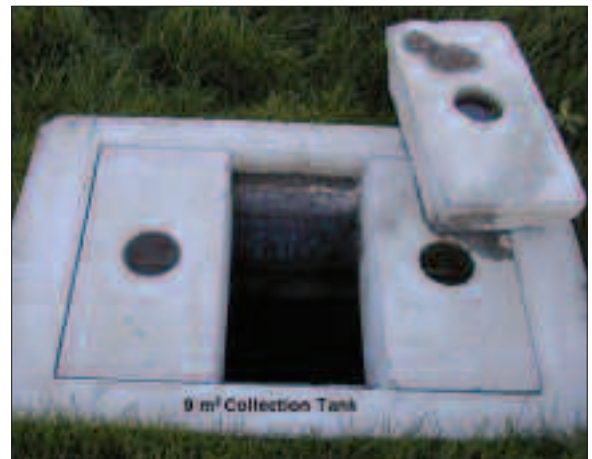
Fig. 2.3 Underground rainwater harvesting 9m 3 storage tank.
