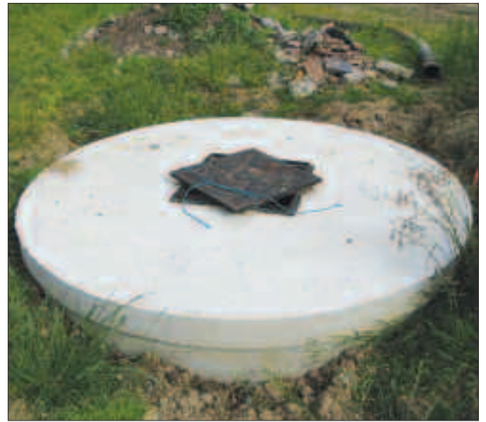
Fig. 3.3 Underground pumping tank.
