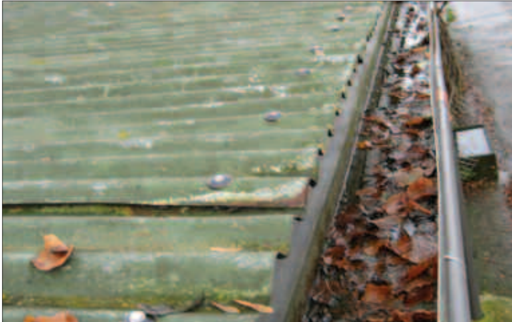
Fig. 3.10 Build up of leaves in gutter leading to failure of custom made filter.
