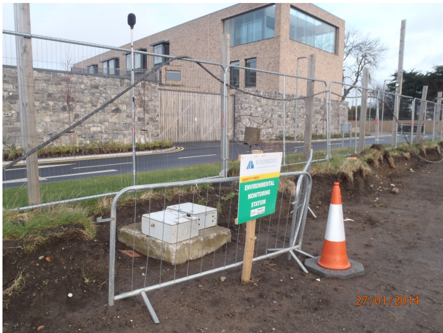
Monitoring Station No 4 @ Energy Building
