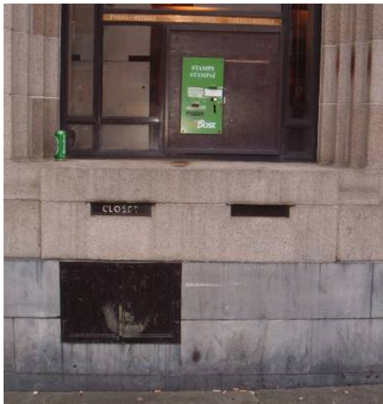
Figure 7/67 Rathmines P.O. 1934; Stamp Dispenser and Redundant Letter Box, Area Showing neglect; Photo, Author, 2007
