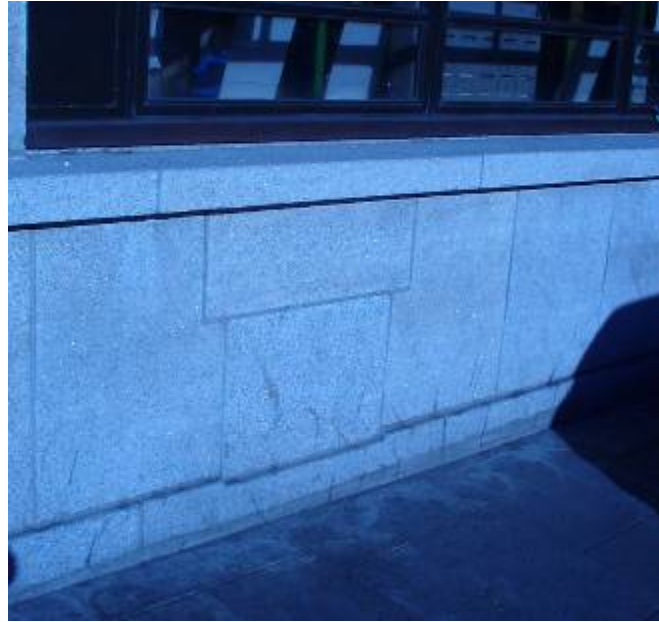
Figure 7/76 – St. Andrew Street P.O. 1947; Blocked up Night Post Box; Photo, Author 2007
