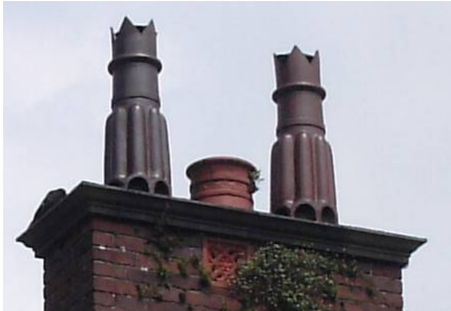
Figure 5/91 – New Ross P.O., c.1903 – Decorative Chimney Pots and Ventilation Grille; Photo, Author 2006.
