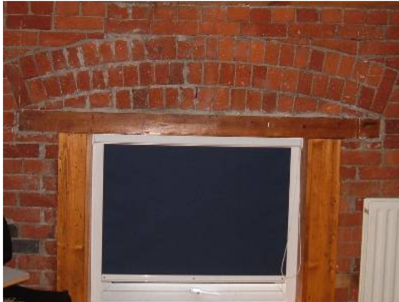
Figure 7/55 – Rathmines Former P.O., c.1883; Original window with timber lintel and brick relieving arch; Photo, Author, Feb 2007
