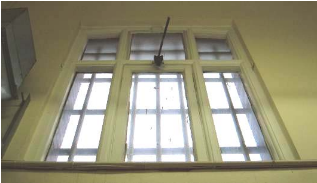
Figure 7/38 – James’s Street Former P.O.; Original Window Frame and Opening mechanism; Photo, Author, 2006
